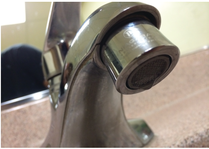
Faucet aerators were added to all faucets in the facility reducing flow rates down to 1.0 gallon per minute.
